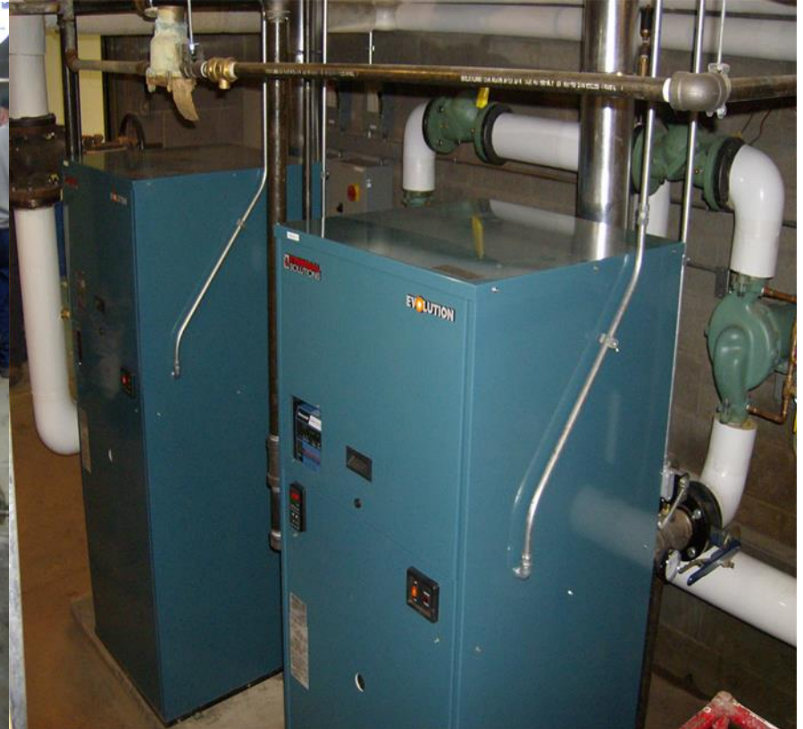
new high efficiency, low emission boiler
