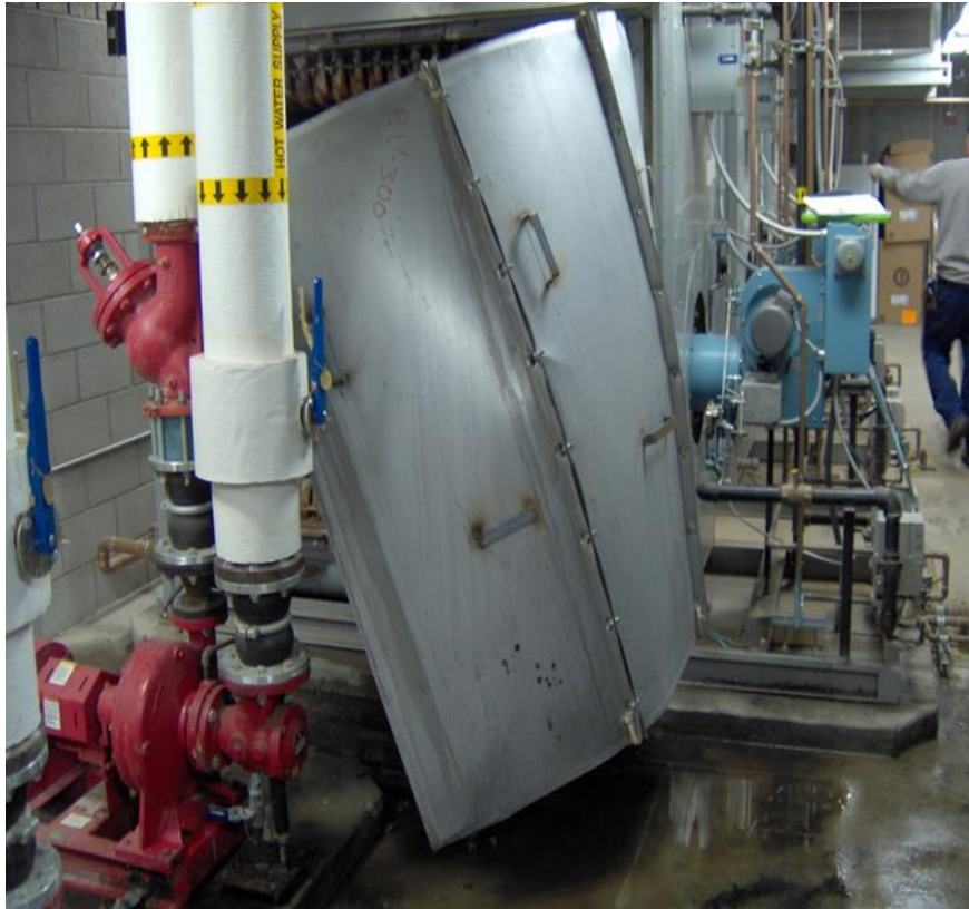
Old boiler after a “hard light”
