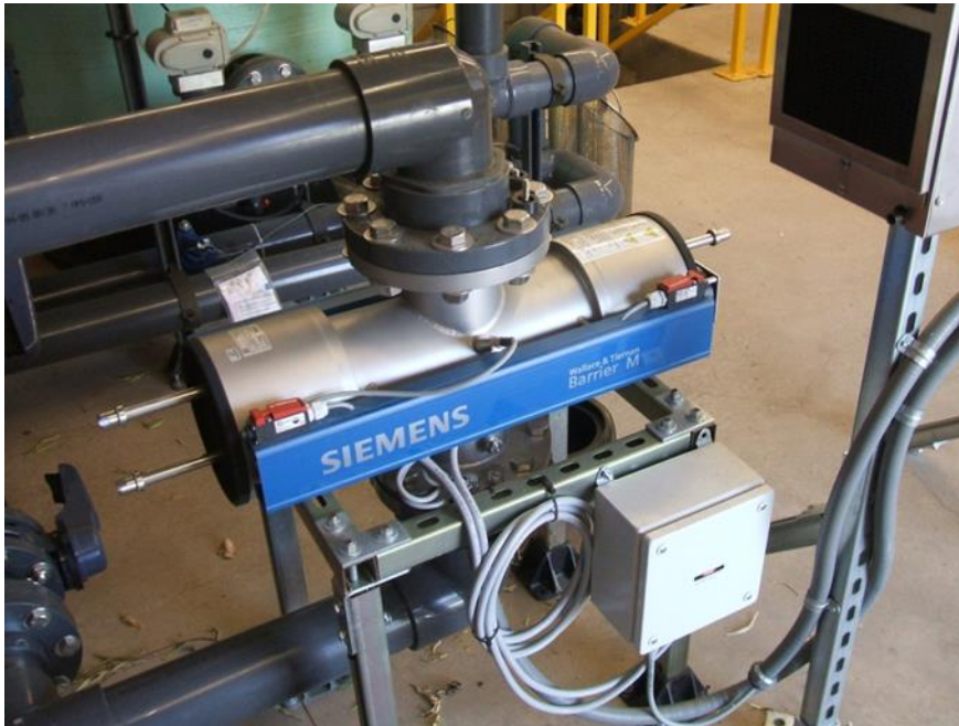
UV Water treatment
